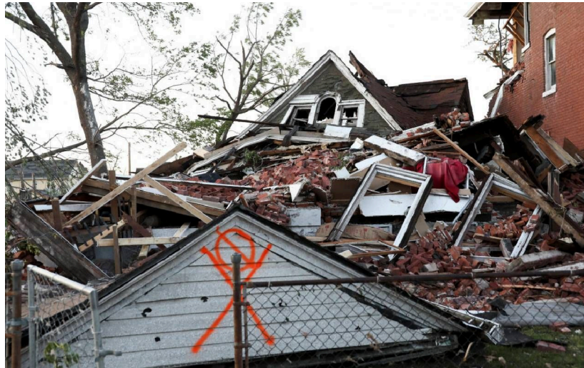
A house lies completely collapsed under a mountain of bricks, after a tornado struck in St. Louis, Missouri, May 16, 2025. | Credit: via PBS NewsHour
